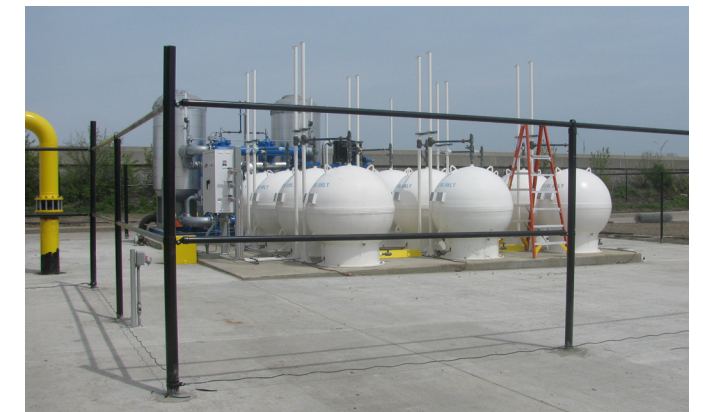
CNG Storage Vessels
