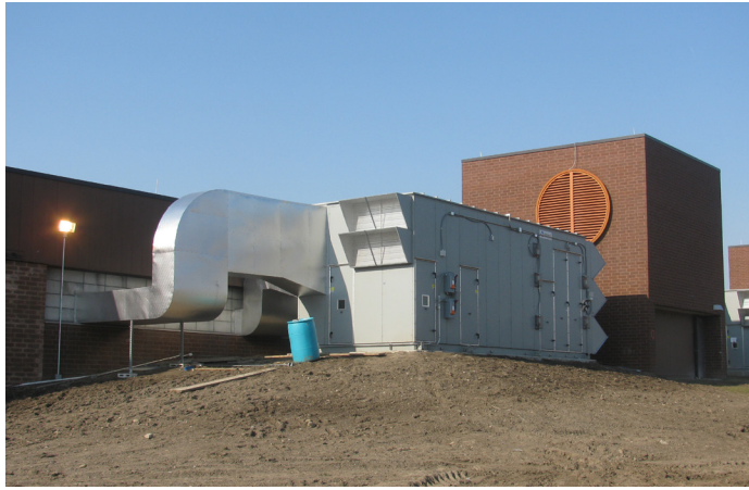
Air Handling Unit
